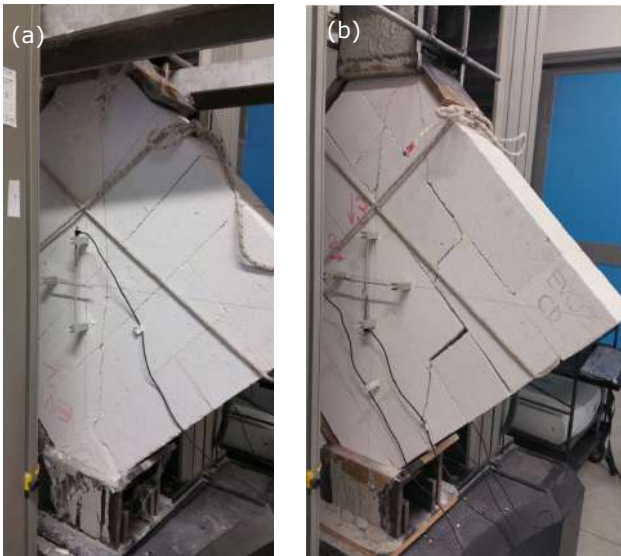
Figure 17 Crack pattern at failure: (a) diagonal crack in the blocks; (b) stepwise diagonal crack pattern in the blocks and in the mortar joints.
