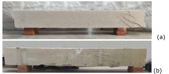
Figure 18 Crack pattern at failure for precast specimens: (a) AAC 20x25-3; (b) AAC 20x25-4.
